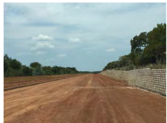
Network Stabilisation Facility
