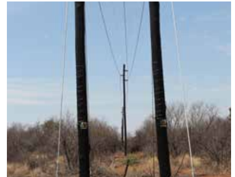
Temporary 32KV power lines, installed to provide power for the construction period, will be replaced by permanent 132KV power lines once the mine is established.
