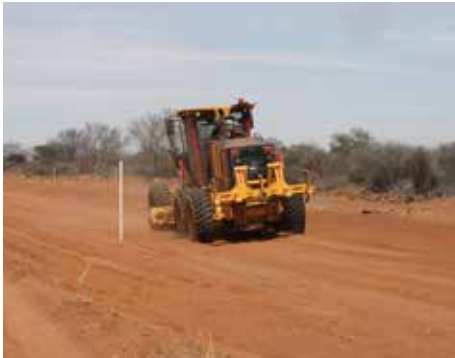
A motor grader levelling the terrace pad at the planned construction camp.
