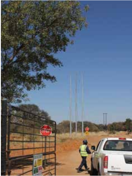
Extended height 22kV powerline poles at Kringgatspruit, chainage 9km, where there is significant fill on the rail line.
