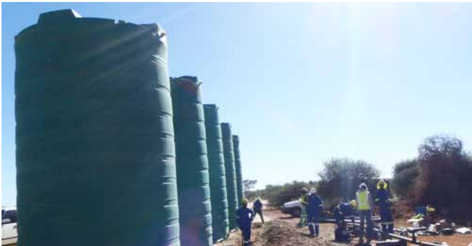
New water tanks at one of the major boreholes on site ZK03.
