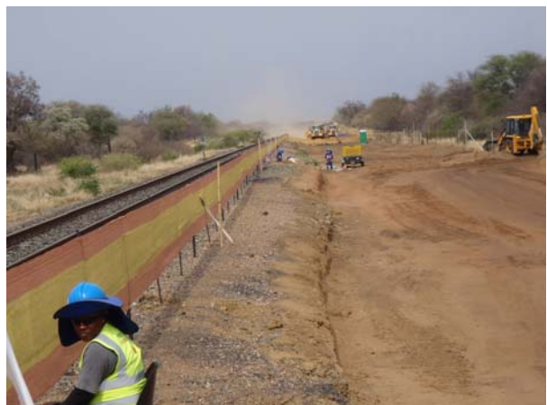
Network Stabilisation Facility
