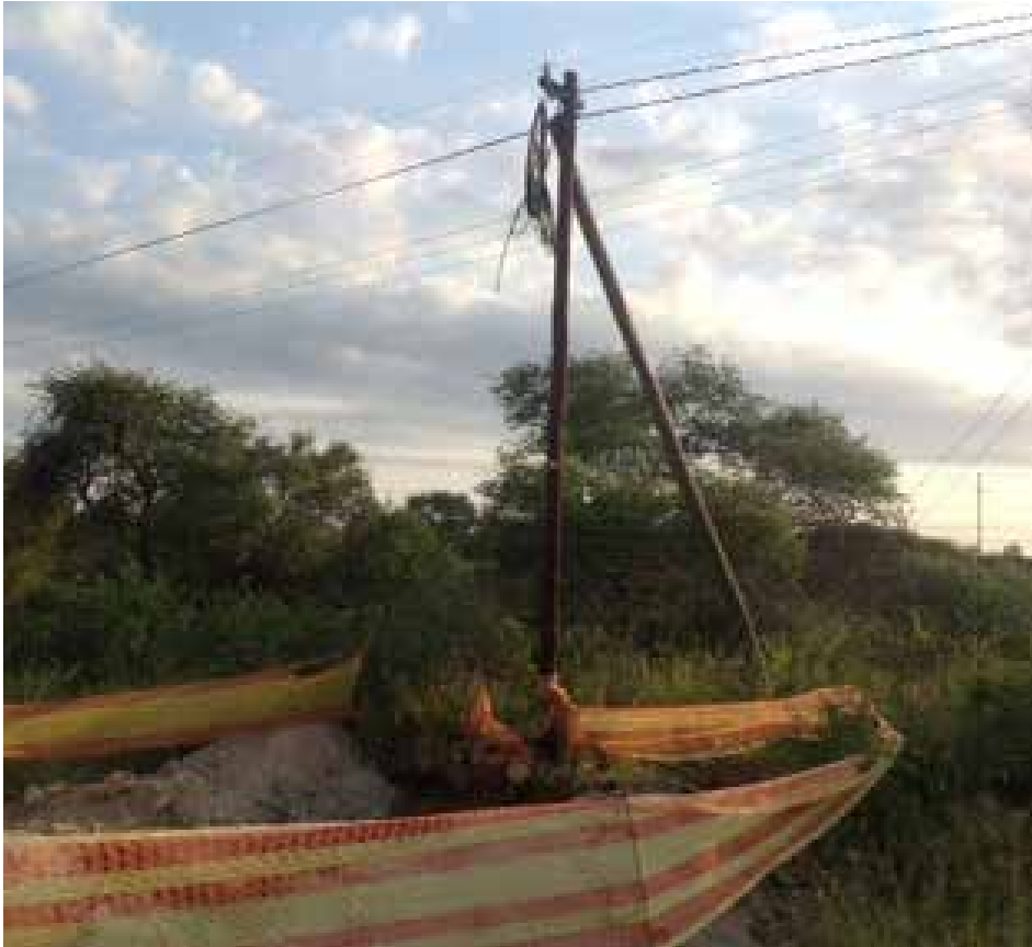
The fibre connection point from the Telkom main line routing towards the mine.
